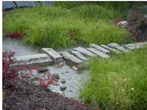
2 Flow Splitters made from granite curbs
